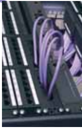
Panel cassette to hub/switch or server
